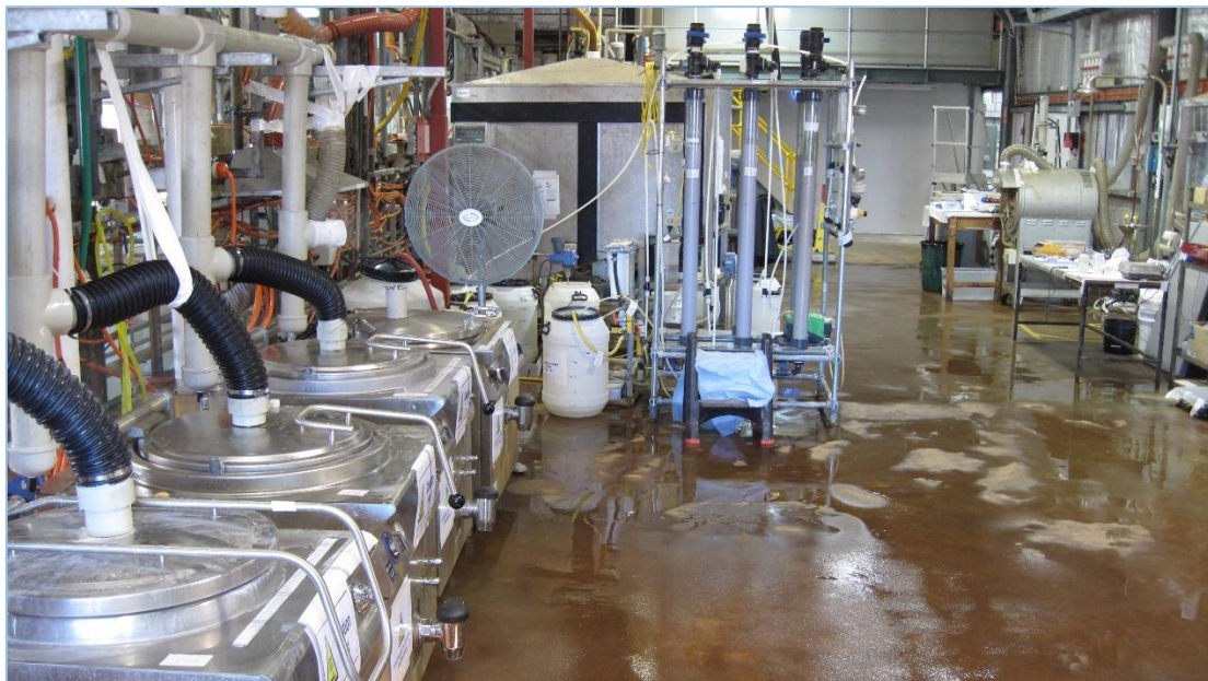
Figure 1 SiLeach™ Pilot Plant trial – Run 1B – lithium carbonate production at ANSTO Minerals pilot testing facility, Lucas Heights, NSW, October 2016.
