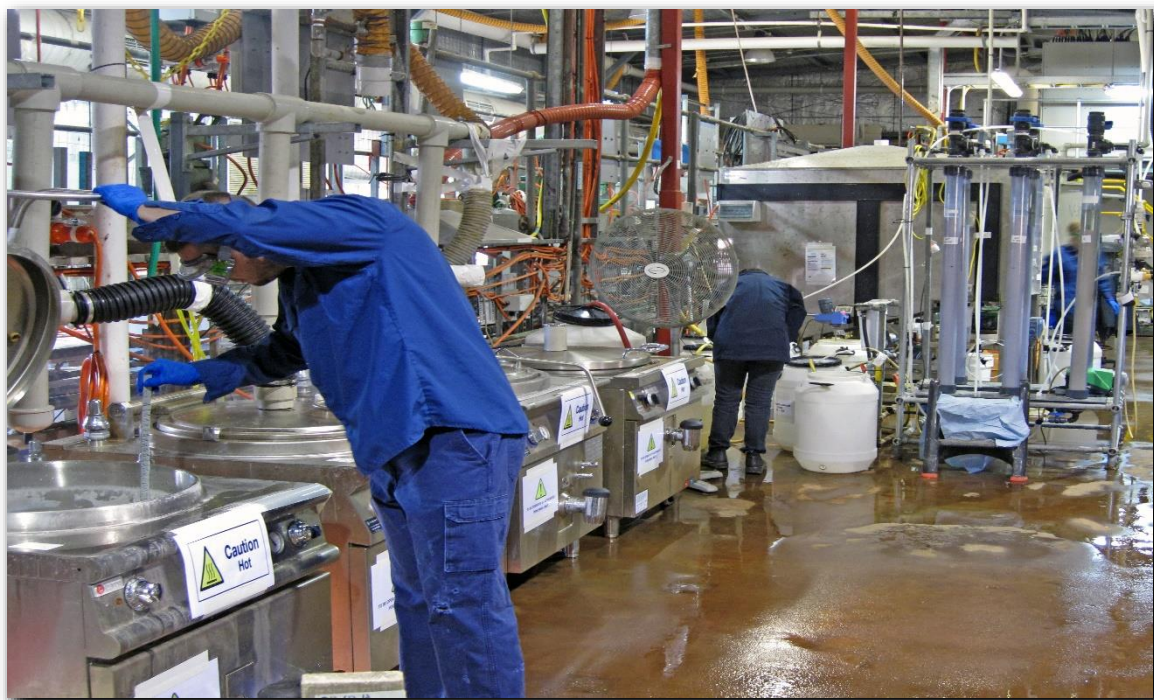
Sileach™ continuous pilot plant operation, ANSTO Minerals, Lucas Heights, NSW.
