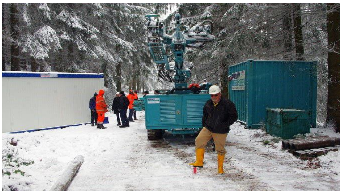
Preparations for drilling at Sadisdorf being overseen by LIT managing director Adrian Griffin.
